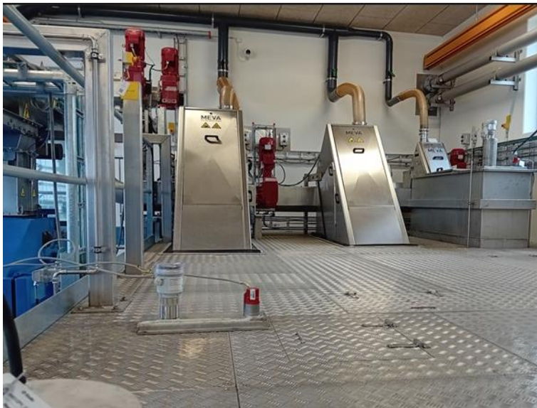
Screens at inlet works
