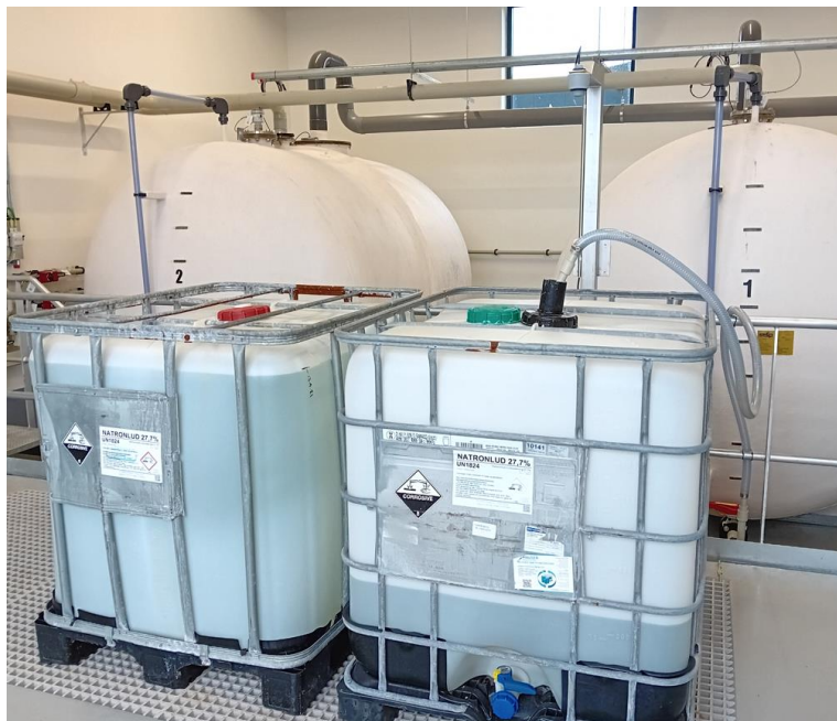
Chemical dosing for P removal
