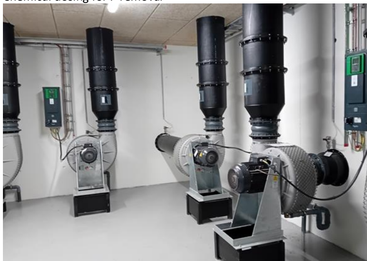
Blowers for aeration lanes
